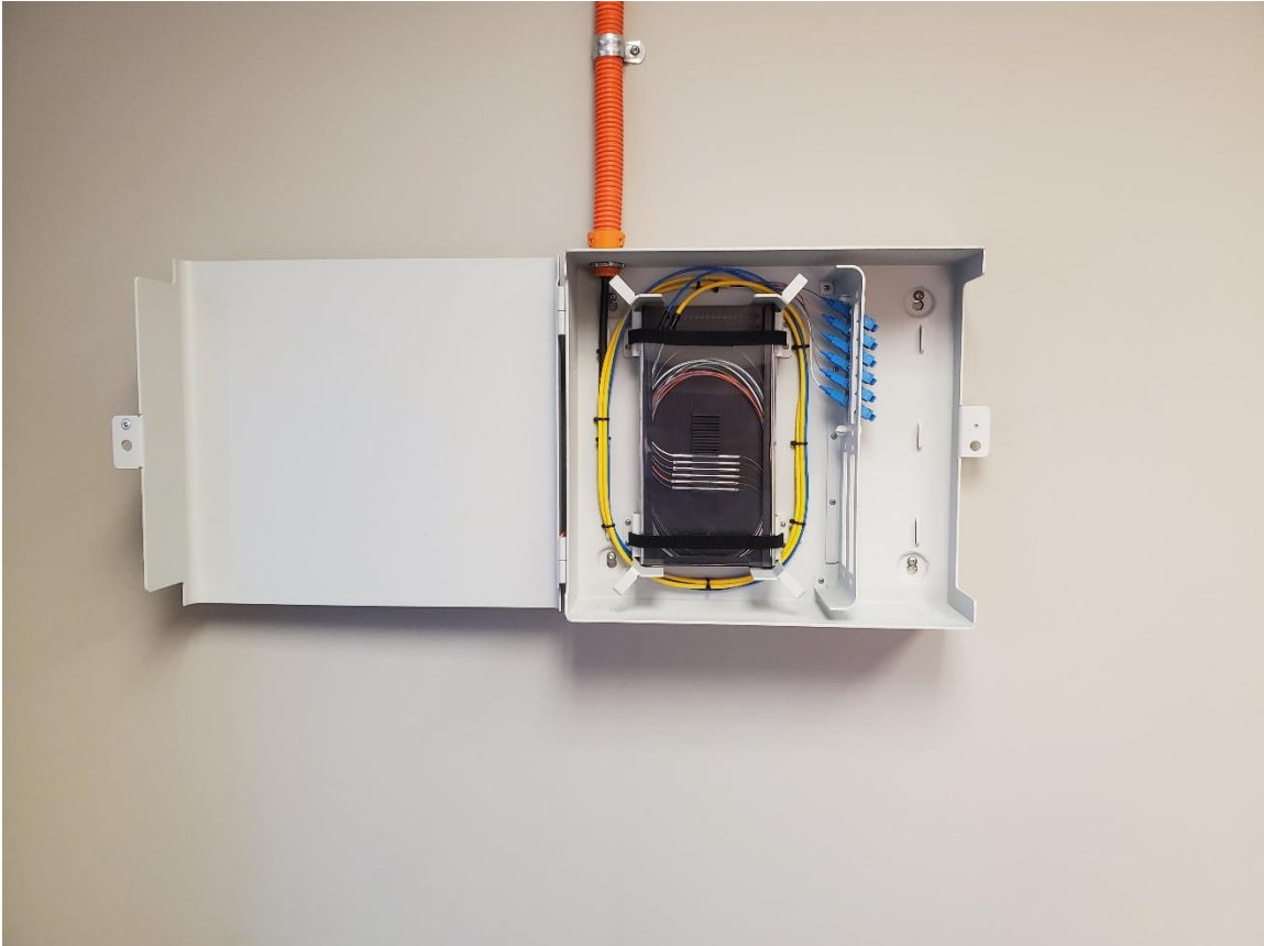
Figure 8. Panel shown with cables neatly affixed to the back panel with splice tray installed.
