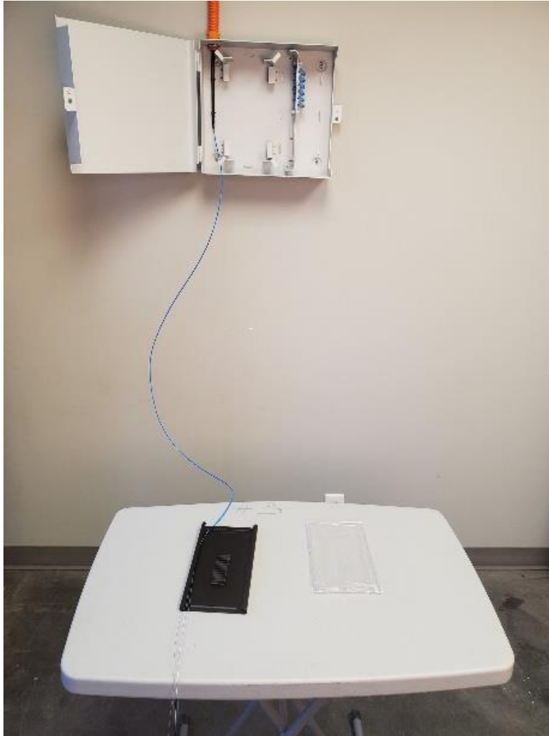
Figure 2. Cable shown with outer jacket stripped back to reach worktable. The outer jacket of the cable is affixed to the back pan using tie straps.
