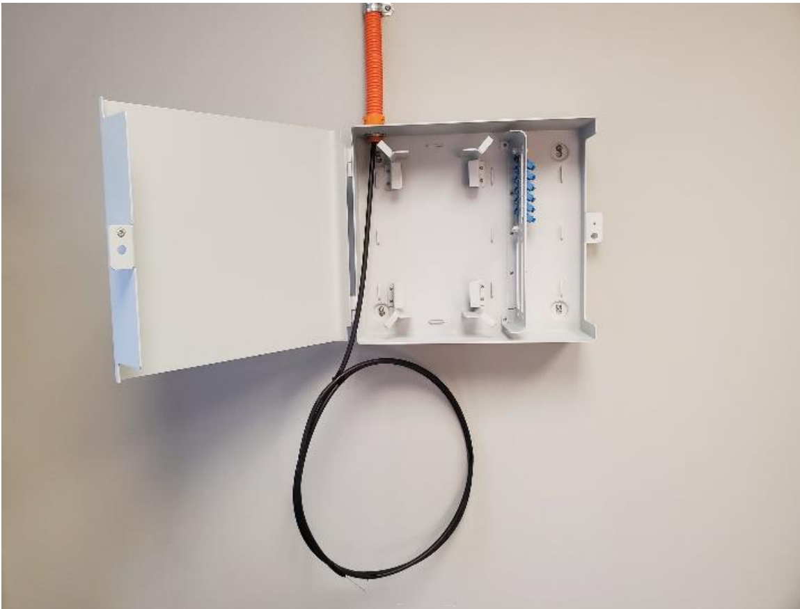
Figure 1. W2 Mid panel shown with entrance cable and one SC/UPC bulkhead adaptor.
